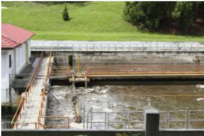
Sewage processing plant
